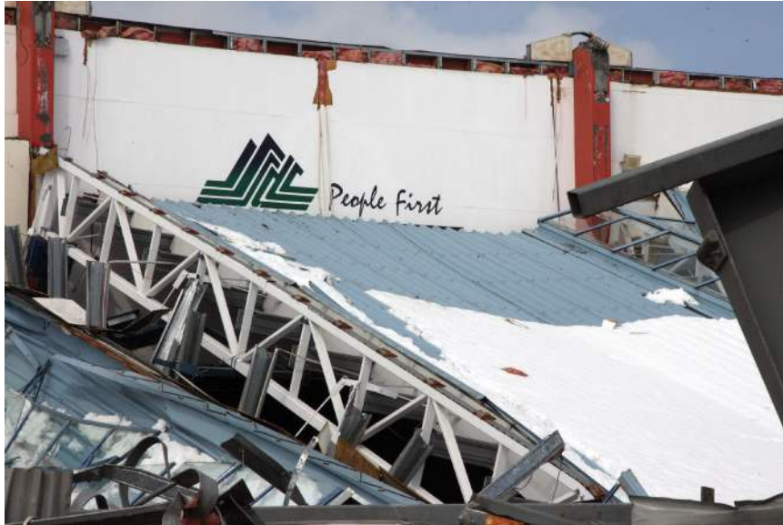
Figure 6: Collapsed roof of Stadium Southland in New Zealand
